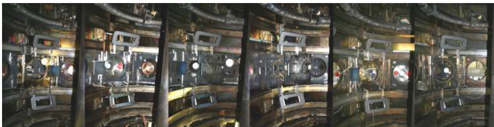
Figure 1.13: The 12 ELM control coils installed in MAST in 2007: schematic (above) and composite of photographs of the coils
