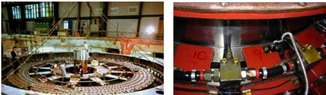
Figure 3.2: A view of the rotor of one of the flywheel generators during original construction (left), in which the surface of the top guide bearing is visible. The photograph on the right, which was taken during the recent inspection and adjustment, clearly shows the top guide bearing pads
