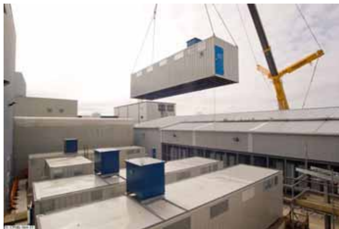
Figure 4.27: One of four modules of the new 60 MVA vertical position control supply (ERFA) being lowered into position in March 2009
