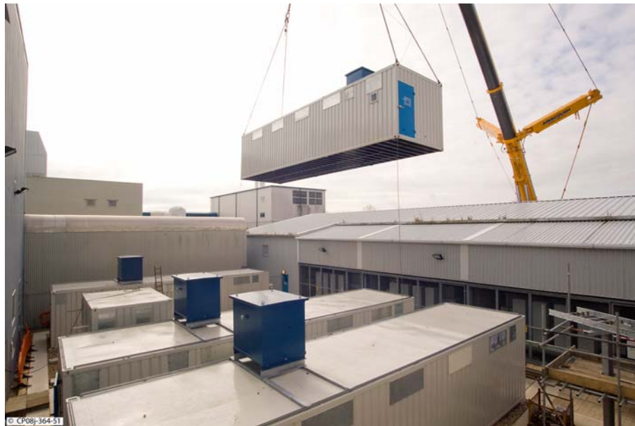
Figure 3.5: One of the six containerised power supply units being craned into final position
