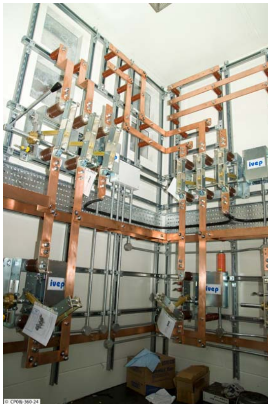
Figure 3.6: Connection box for selecting ERFA or FRFA operation of radial field circuit
